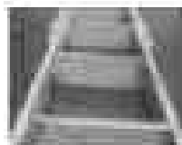
Crack on the rung
