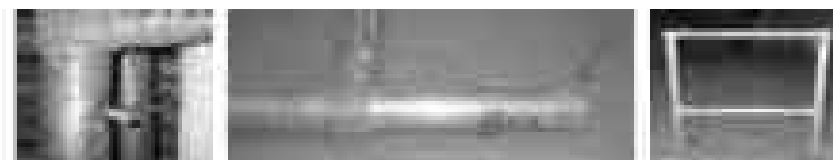
Broken flanges on the lateral frame
