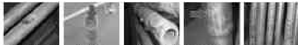
Rusty on lateral frame
